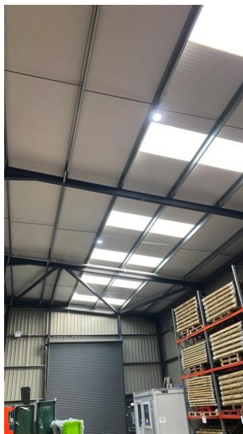
Figure 3-2 New warehouse lighting and roof lights
